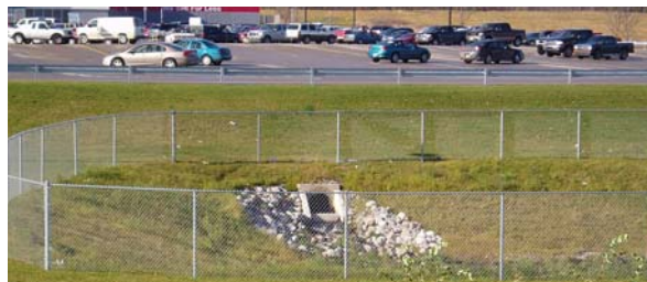
Retention Pond Used by a retailer along the Business Loop
